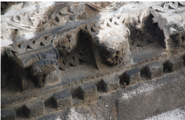
Fig. 9. Peristyle, cornice of the Prothyron gable, detail before restoration (photo: Croatian Conservation Institute)
